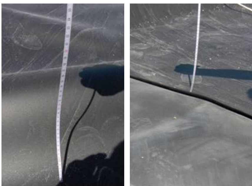
FIGURE 7 - Measurement of shape deformation of geomembrane due to delay of concrete covering.
