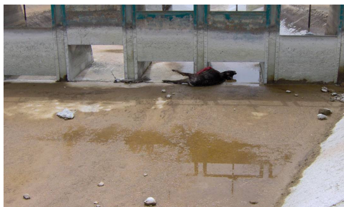
Figure 6. An animal stuck to a gate of a hydraulic structure at Urfa main canal.
