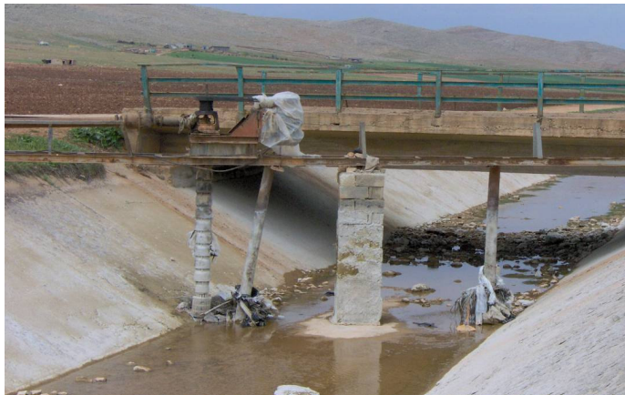
Figure 5. Unauthorized water outlet at Urfa main canal.
