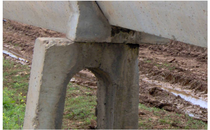
Figure 4. Sliding of supports at canalette.
